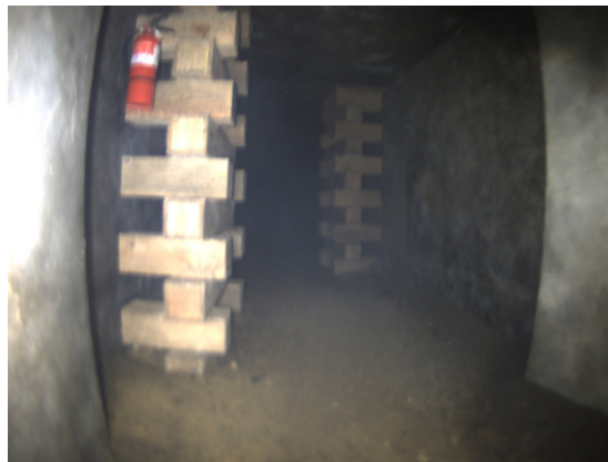
Figure 49. Missed fire extinguisher only seen for a few frames by the right camera of D01.
