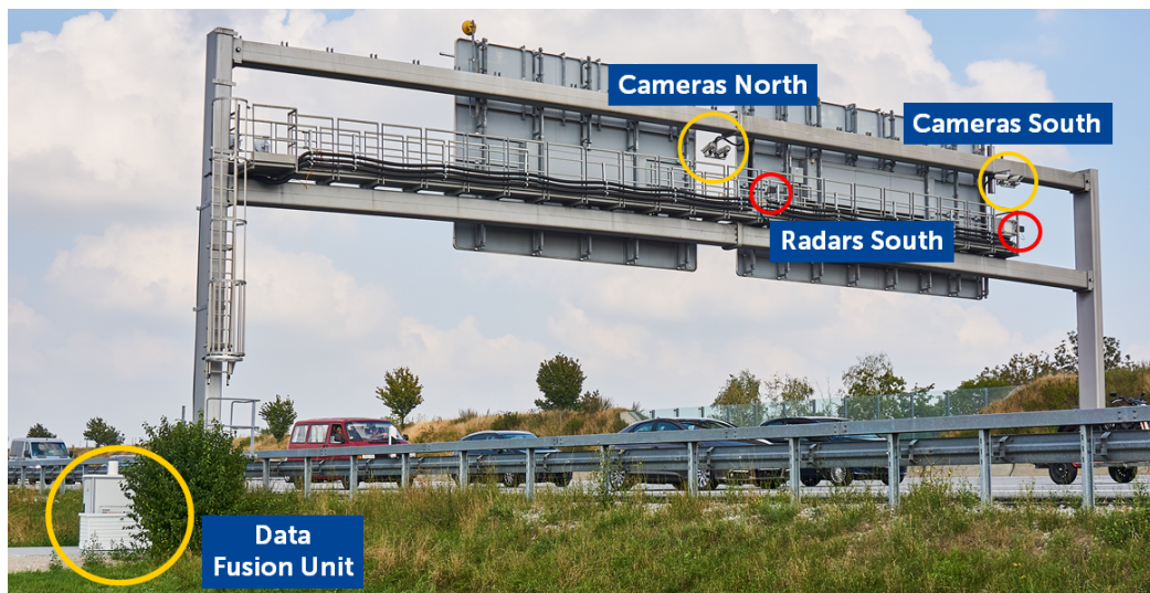
Figure 1. One of the Providentia measurement points on the A9 highway. The two radars directed towards the north are installed on the other side of the gantry bridge and are therefore not visible from this perspective.
